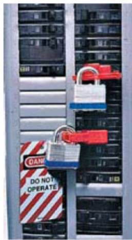
Danger tagged circuit breaker locking off devices
